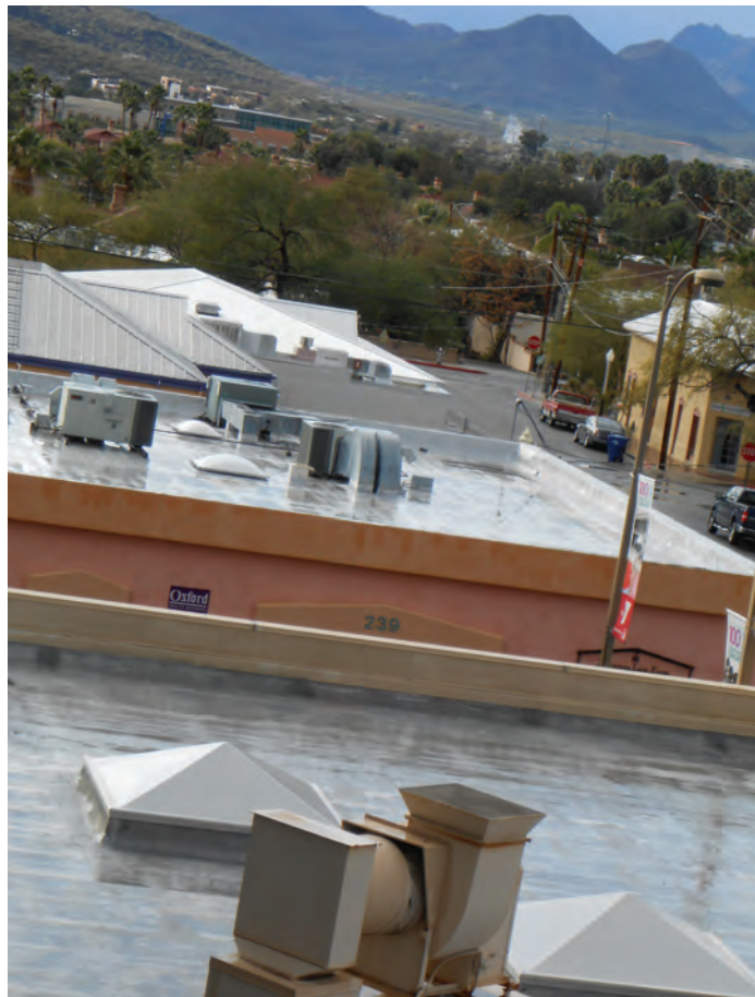
Typical rooftop equipment.
