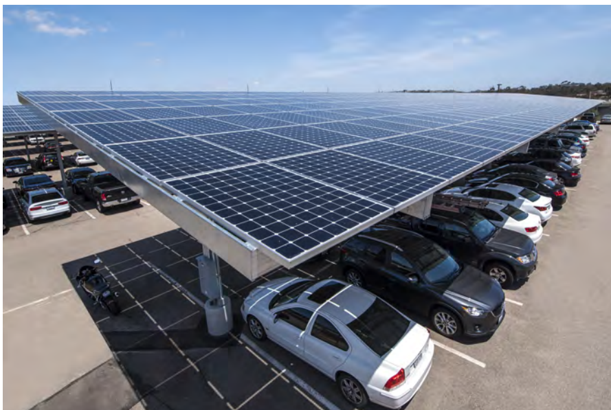
An example of an elevated PV support structure.
