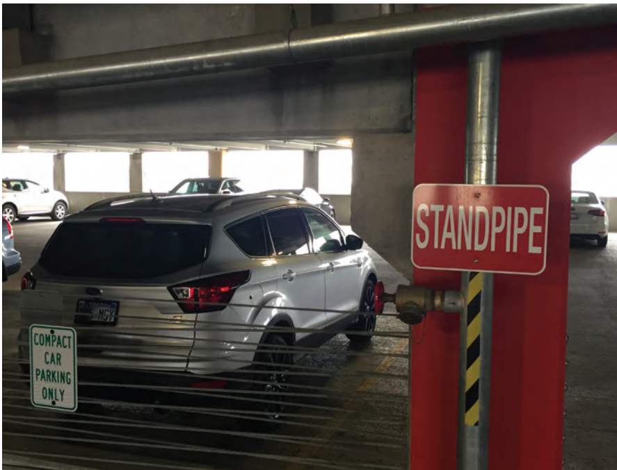
Class I standpipe in parking garage.
