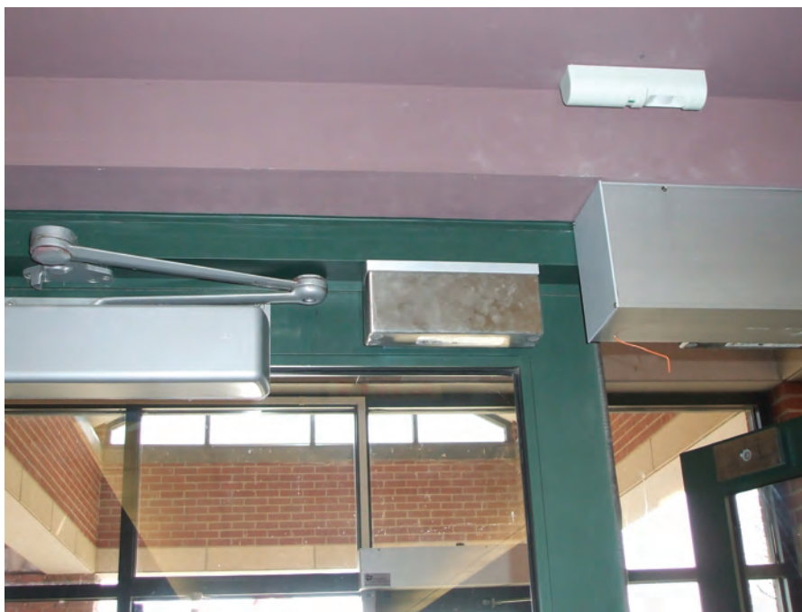
Door closer and electromagnetic lock projecting into door height.
