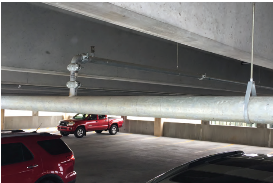
Sprinklered open parking garage.
