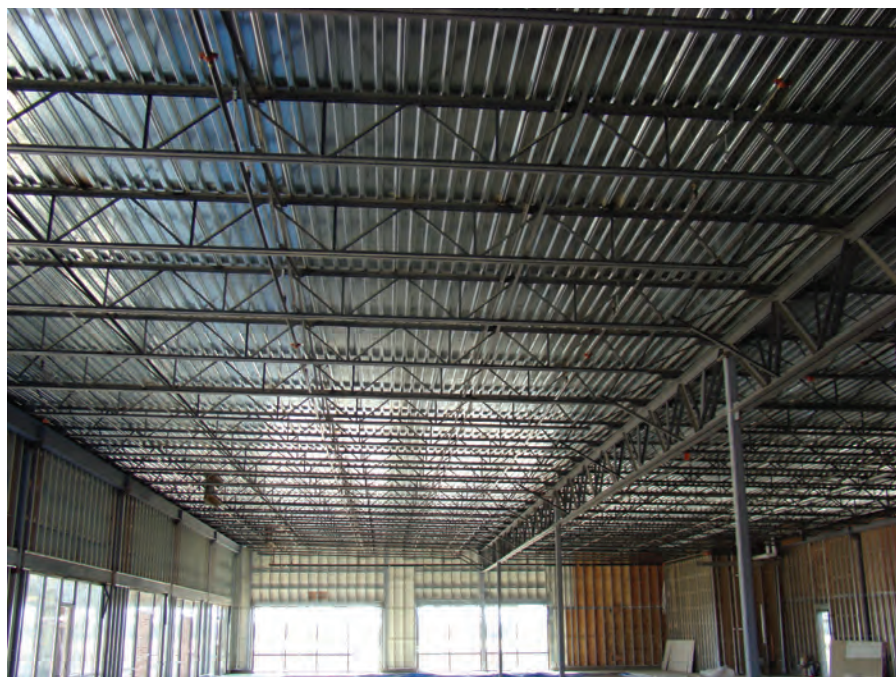
Columns and girder trusses form the primary structural frame in a roof; trusses are considered secondary structural members.
