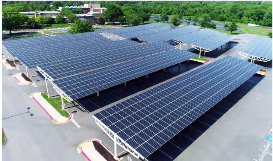
Elevated photovoltaic support structure.
