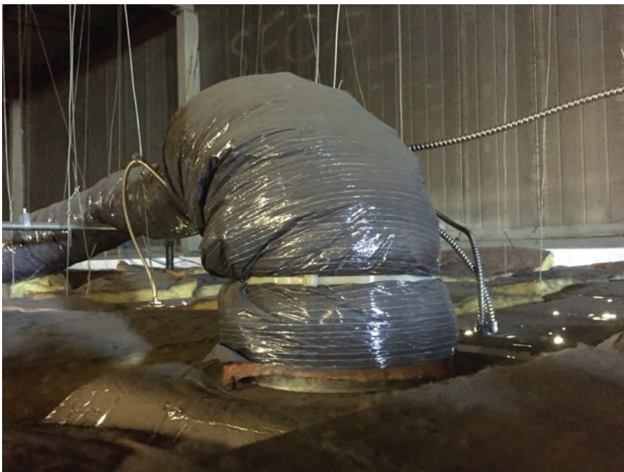
Flex connector to ceiling diffuser.
