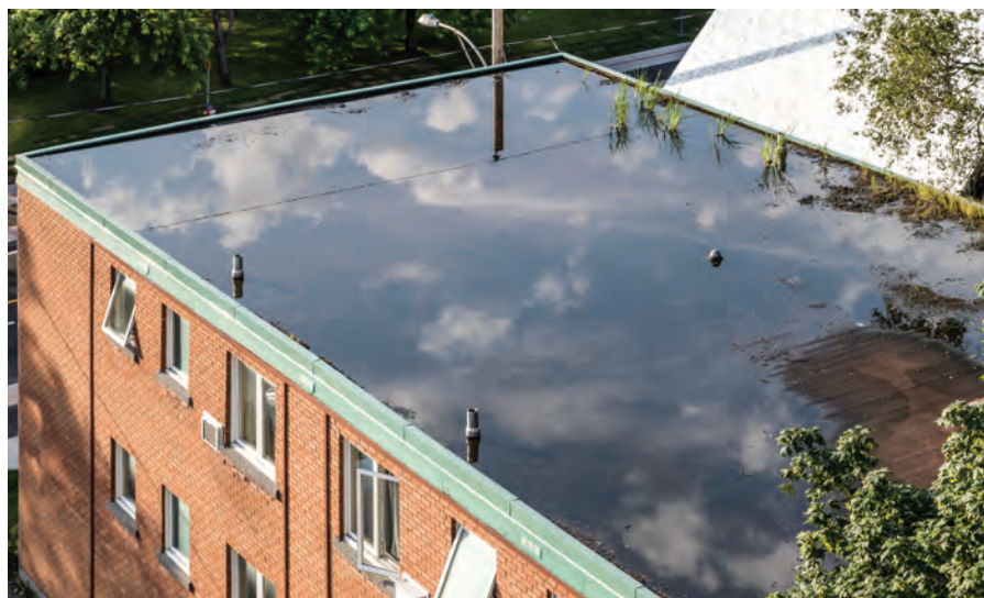
Frequently flooded roof.
