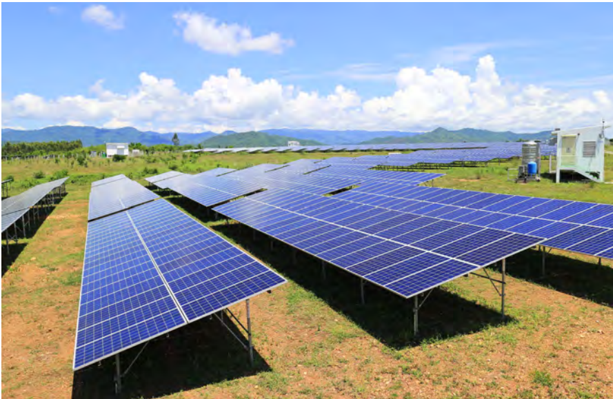
Ground-mounted photovoltaic panel system.
