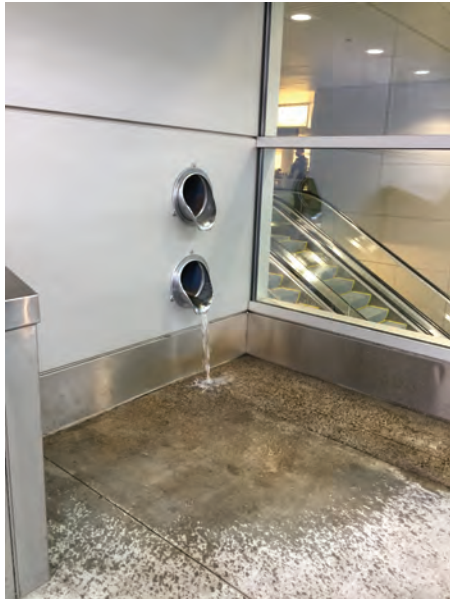
Secondary drainage system outflow.
