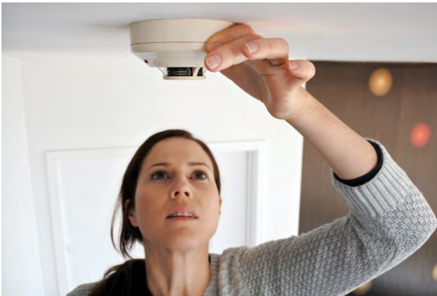
A ceiling-mounted automatic smoke detector.
