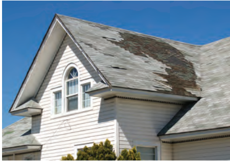
Roof cladding damage.
