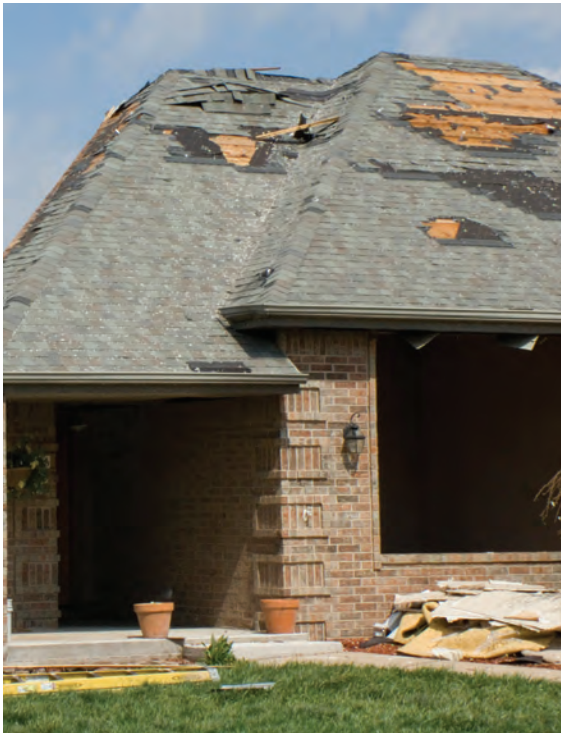
Wind damage to roof and walls.
