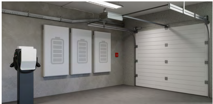
An example of ESS located in an attached garage.
