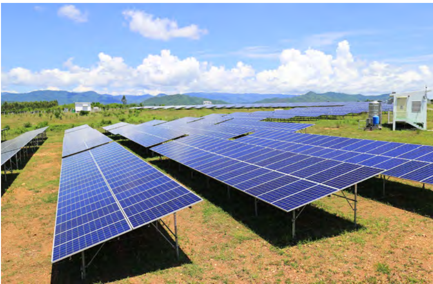
A ground-mounted photovoltaic system.
