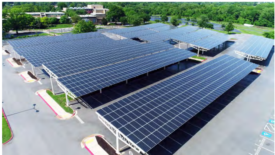
A photovoltaic support structure.
