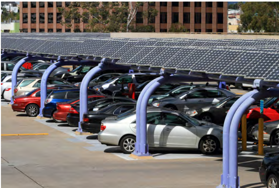
An elevated photovoltaic support structure used in a parking facility.
