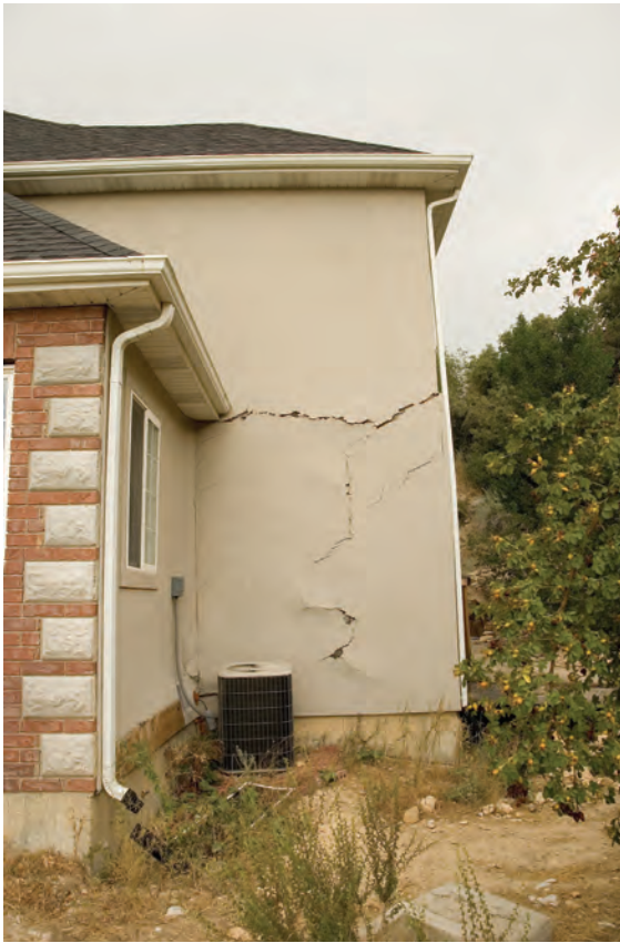
Damage due to ground movement.
