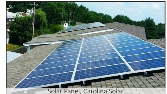
Solar Panel, Carolina Solar
