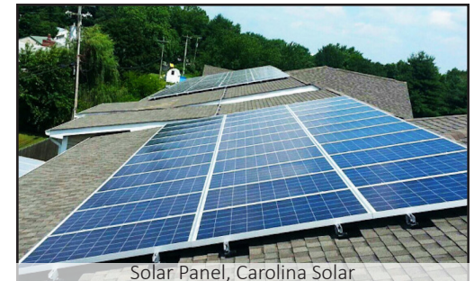
Solar Panel, Carolina Solar
