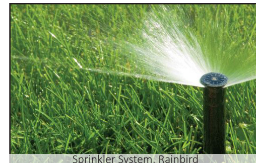
Sprinkler System, Rainbird
