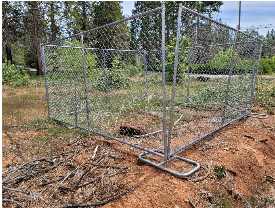
Photograph 7, view facing southeast: Septic at 1623 Cypress Lane, APN 050-140-161.
