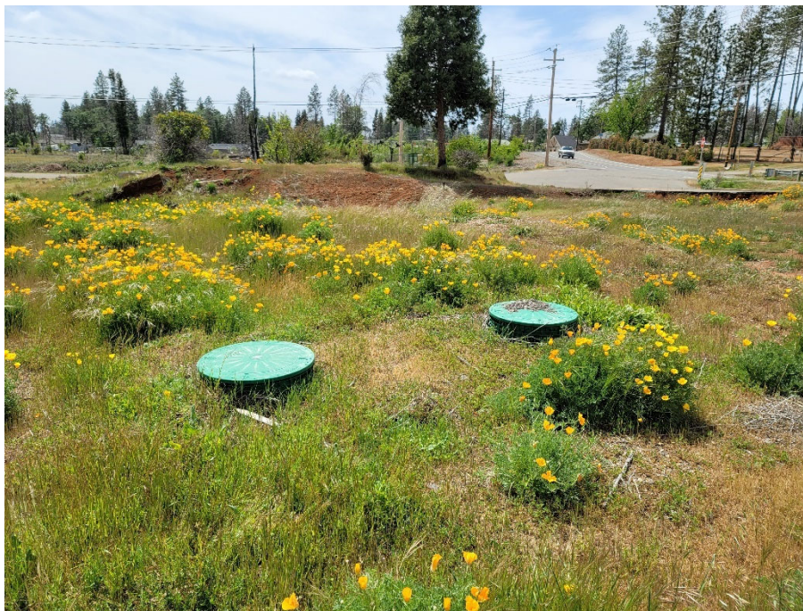
Photograph 4, view facing south: Septic at 6900 Clark Road, APN 050-140-160.
