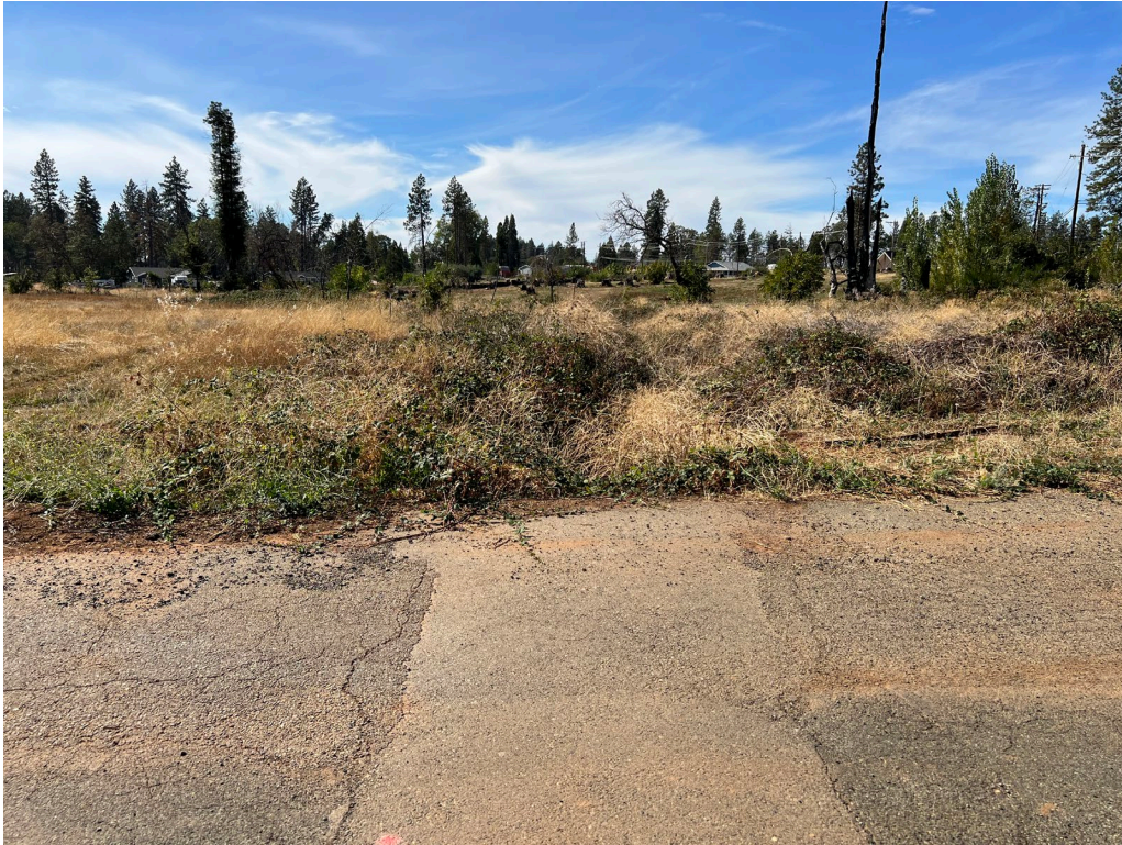
PP5: Standing over the Cypress Ln culvert of Stream Channel 1, looking southwest
