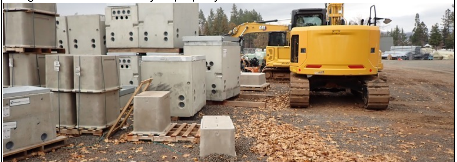
Image 3. Equipment observed on the subject property.
