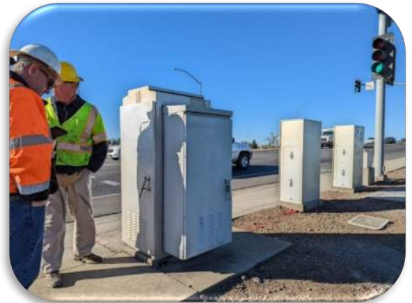
Exhibit 6: Signal Cabinet on Skyway
