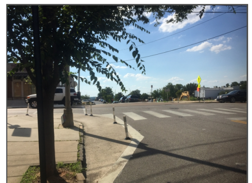
Interim curb extensions can be installed using pavement markings and flexible delineator posts as shown in this
