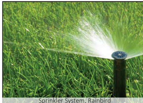
Sprinkler System, Rainbird
