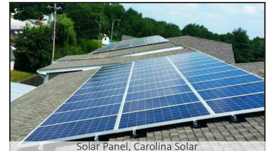
Solar Panel, Carolina Solar
