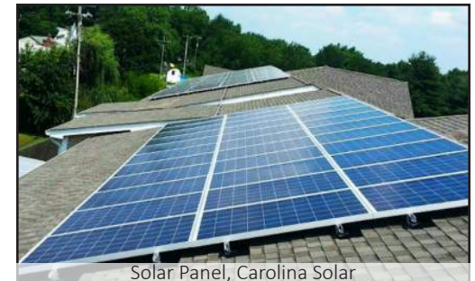
Solar Panel, Carolina Solar
