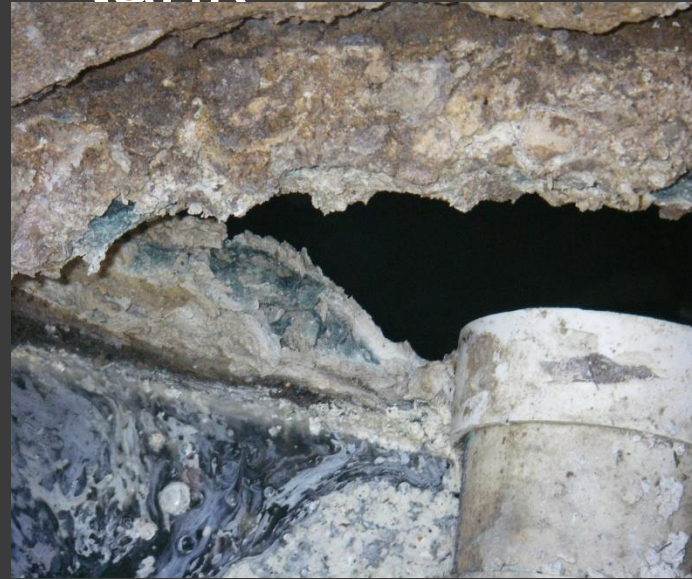
Corrosion inside tank
